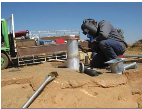
WFTO Hand Pump Technician, Lot Ncube, is pictured welding a new pedestal stand flange at the Chisankane Market hand pump
